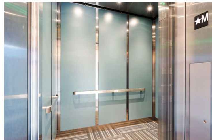
COMMON AREA - ELEVATOR
